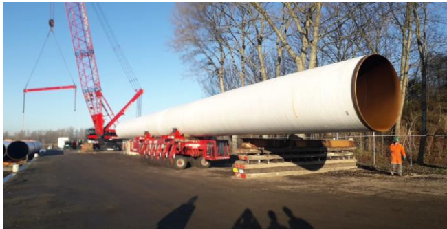
Figure 4-13 Bogmat set-up 'Kerksloot' to increase storage capacity
