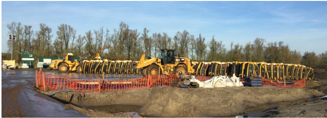
Figure 4-36 PipeSak storage area
