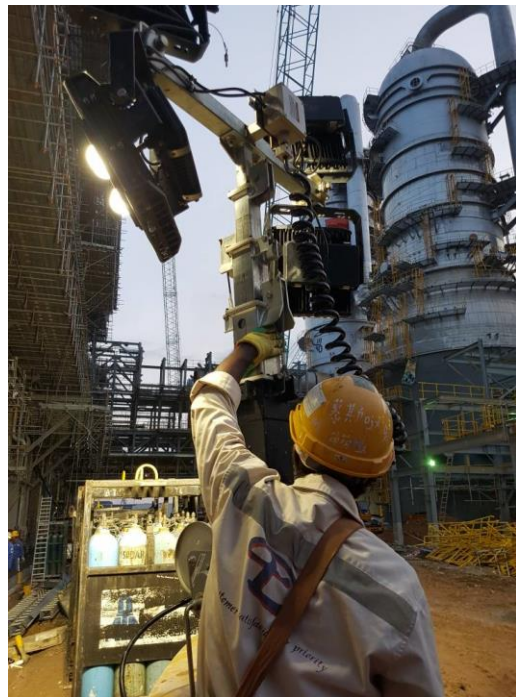
IP grasped the cable and pulled to release the jam
