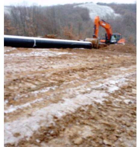
The moment the excavator stopped the pipe
