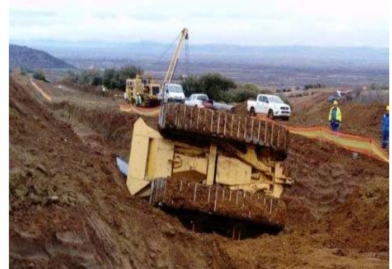
Conditions After the incident.
