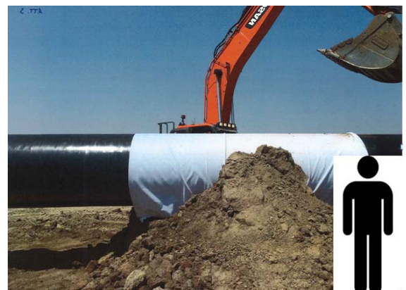
Recreation of the position of the excavator and worker at the time of the incident
