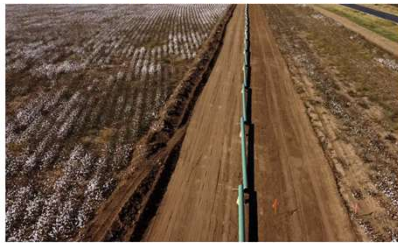
Pipes sit in a cotton field waiting to be installed for new oil pipelines in Lenoir, Texas. Photograph: David Goldman/AP
