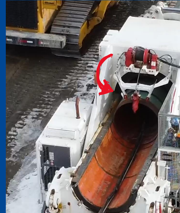
Bending Safe Hook Support is moved down onto the pipe for hook release
