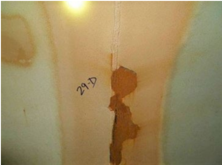
Failed internal field joint coating – a common occurrence.
