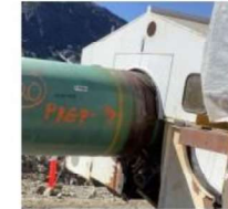
Closer view of the pipe and shack following the incident.
