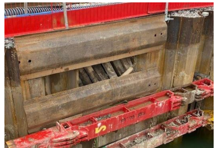
Timbers showing movement following heavy rain
